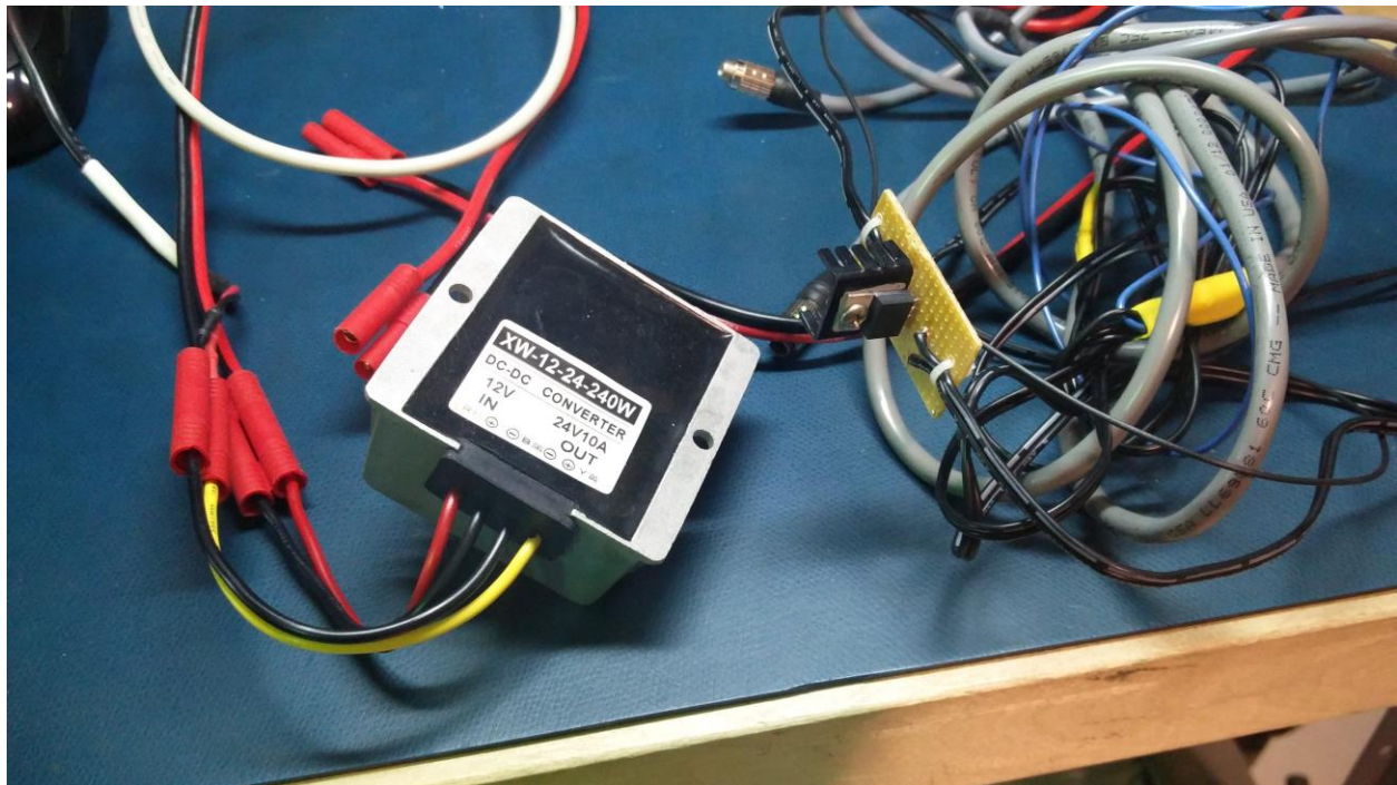
Fig. 3: New and improved power supply setup for the sensors
