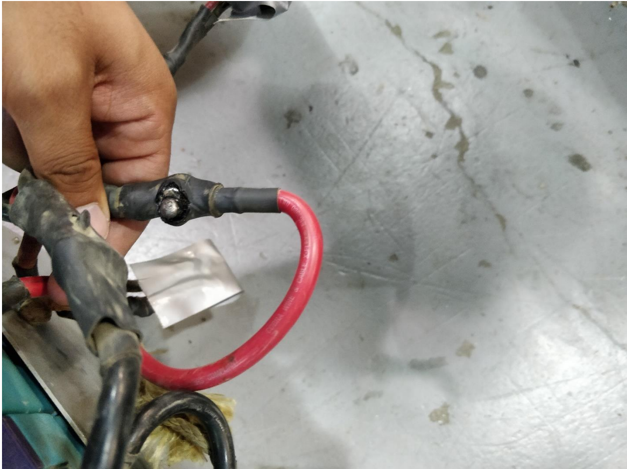
Figure 2 The tear I identified on the battery cable
