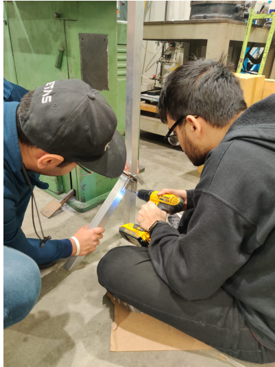
Figure 2: Manufacturing of one of the infrastructure mounts
