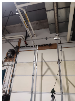
Figure 3: Infrastructure units ready with camera mounts
